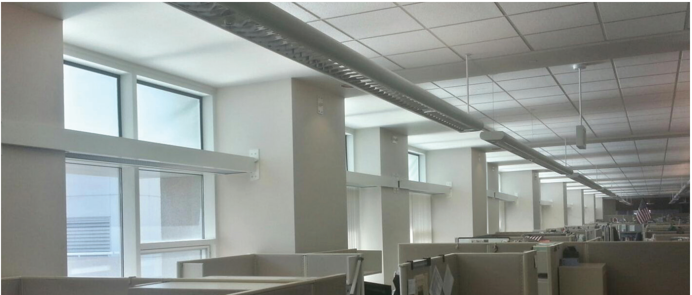
3M™ Daylight Redirecting Film installed in Clerestory Glass — Sacramento, CA
