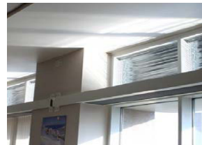
Daylight Redirecting Blinds (Daylighting Zone)
